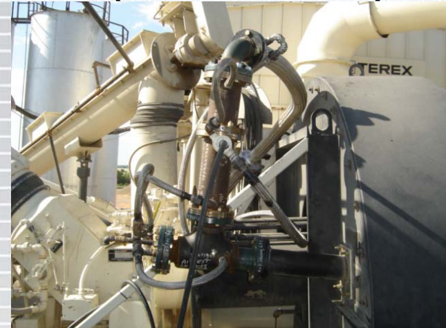
Mixing chamber and piping installed (no insulation)
